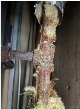
Figure 7 Old riser take off
