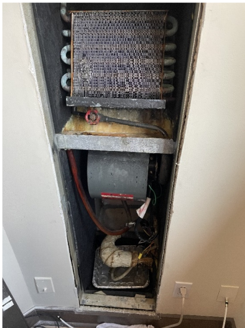
Figure 8 Fan-coil Unit Before
