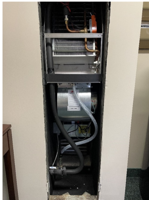
Figure 9 Fan-coil unit After
