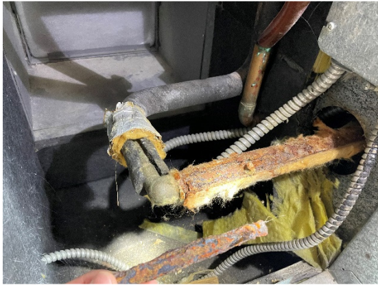
Figure 3 Corroded run-out pipes
