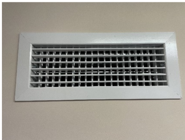
Figure 10 new fancoil supply grille
